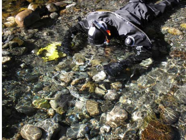
Figure 8. A redd with 6 buckets and a layer of clean gravel being hand placed over the top of the buckets.
